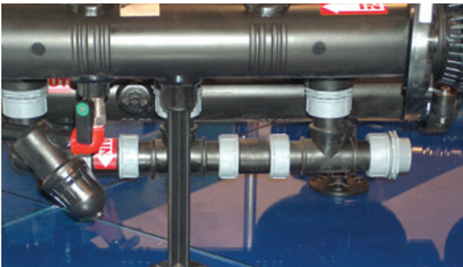
Filtration battery flushing manifold
